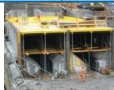
Desander plant Burglauenen
